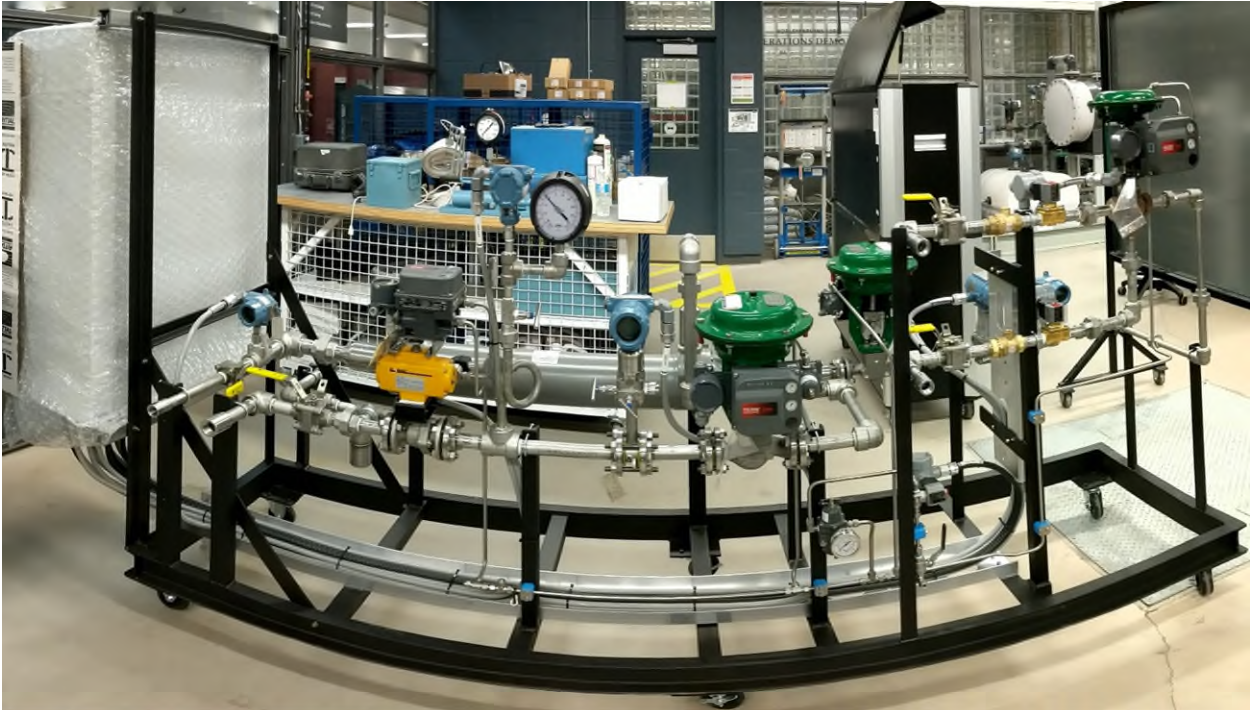
Figure 69: Full plant, inlet and outlet side
