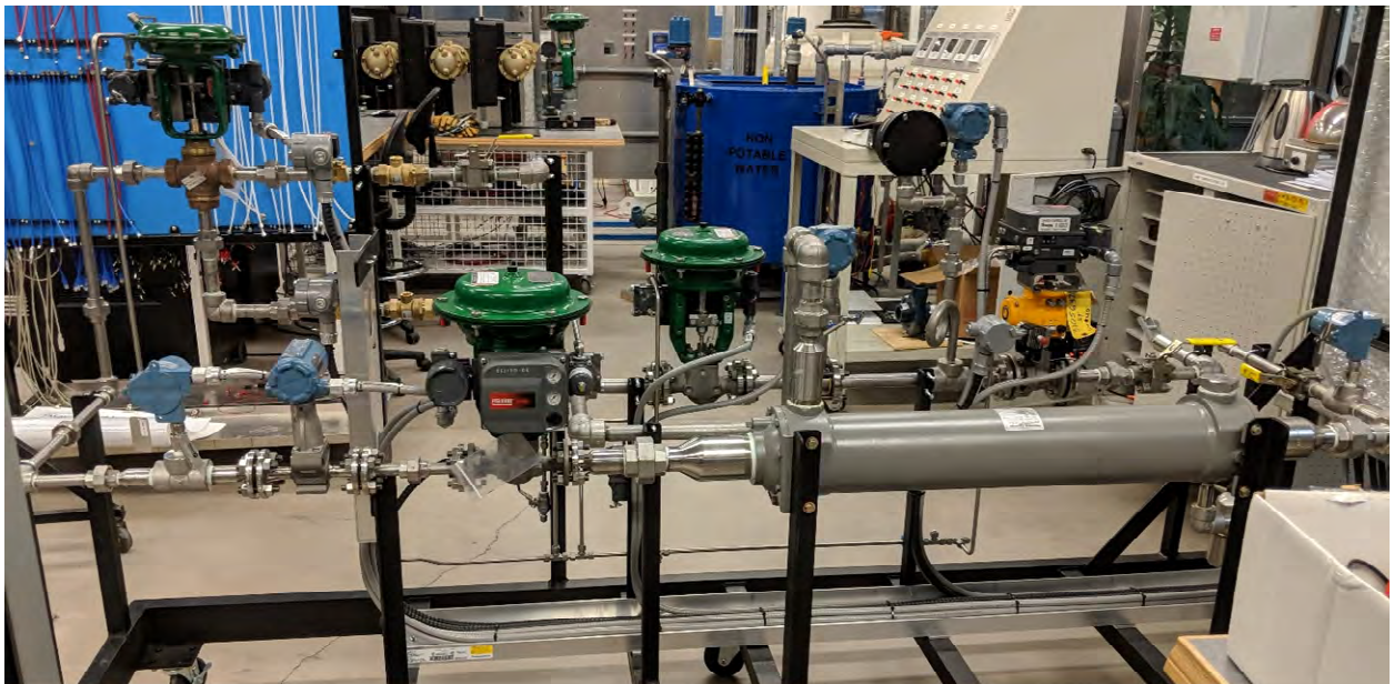
Figure 68: Full plant, Heat Exchanger side
