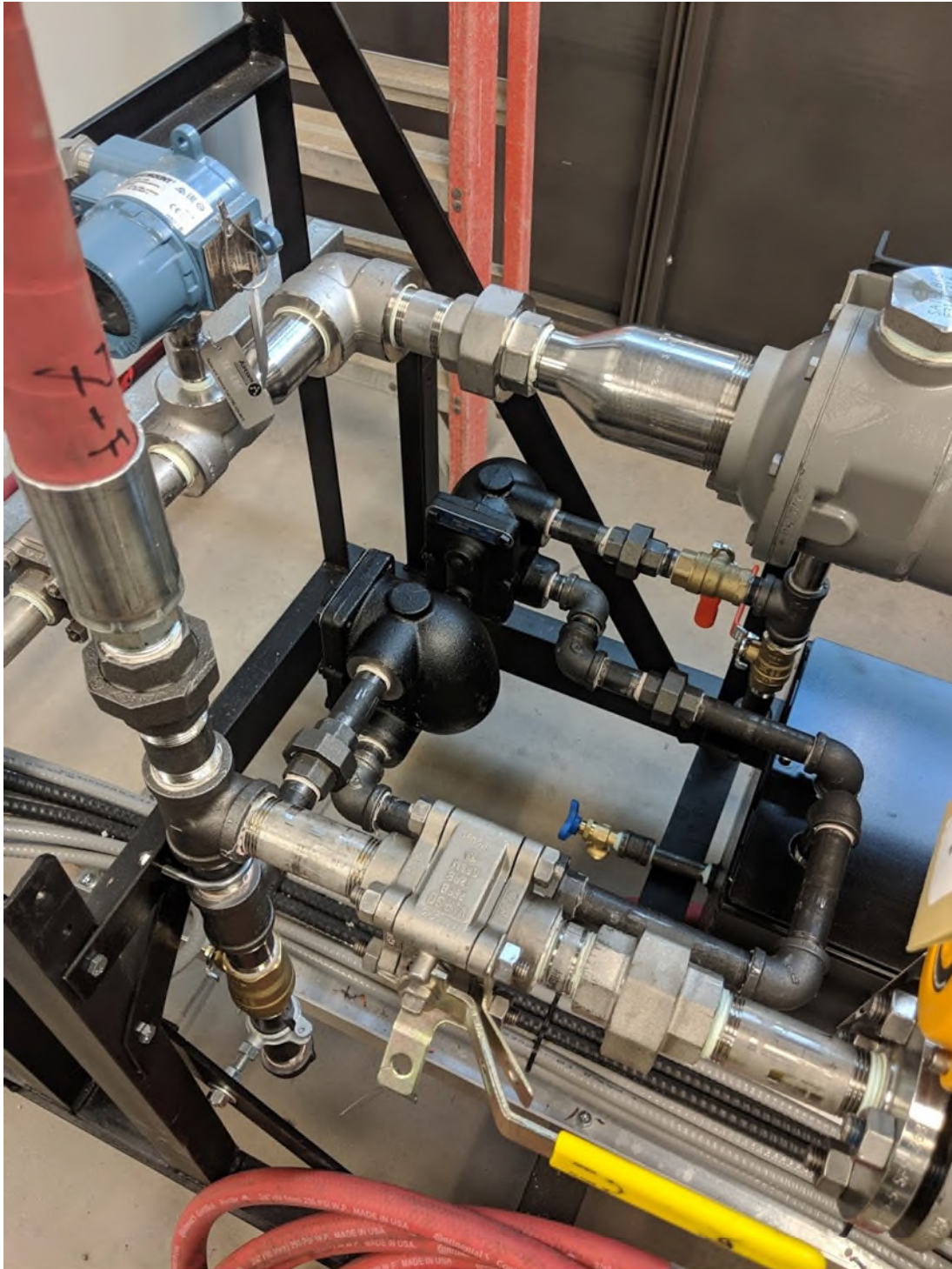
Figure 72: Plant condensate traps
