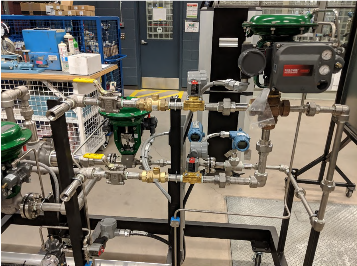
Figure 70: Plant Process Inlet Lines
